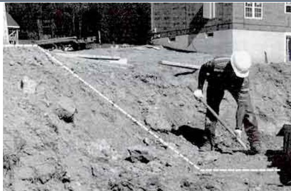
Figure 20. The dotted line shows the profile of this excavation, as it was sloped at 1\frac{1}{2} : 1 . Usually residential excavations are type C soil and will require such a slope. The spoils pile is at least 2 feet back from the edge of the excavation.
