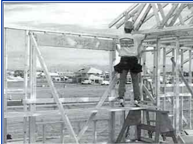
Figure 14. This worker uses a recognized safe work practice by standing on a work platform to secure the end of the roof truss.
