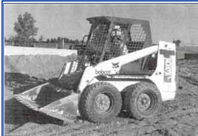
Figure 22. This worker has been properly trained to operate this piece of equipment, and it is equipped with the appropriate safety devices.
