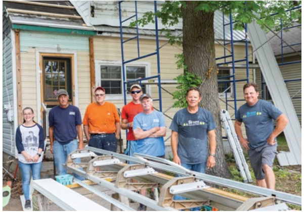
A combination of volunteers, Habitat staff, subcontractors, and homeowners completing Sweat Equity hours are all part of the home repair efforts.
